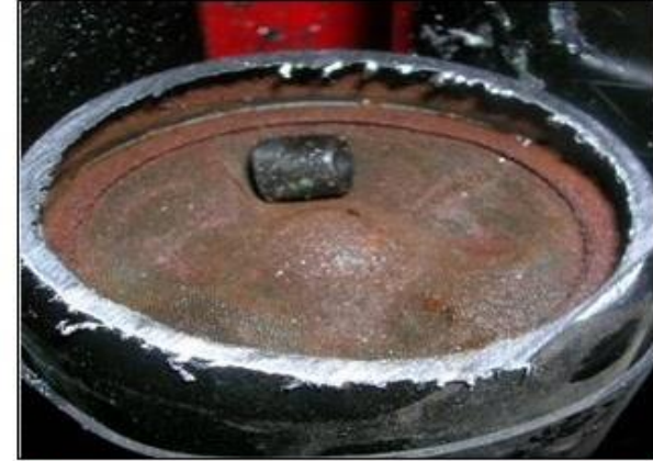
Accum. baffle Rusty & deform
