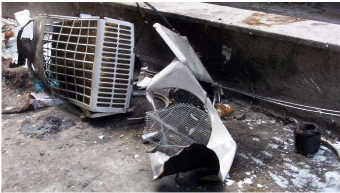
An outdoor unit was severely damaged
